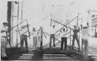
Management Process personnel shown dismantling a scaffold in the HDS West Area include Vice President Per Nord (c), acting Process Manager Joaquin Croes (3rd right) and HDS Division Supt. Julio Curiel (2nd l).
